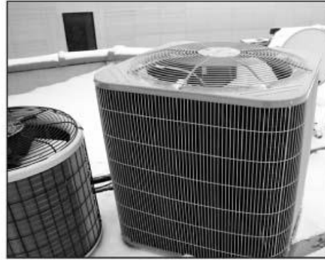
Air conditioning systems
